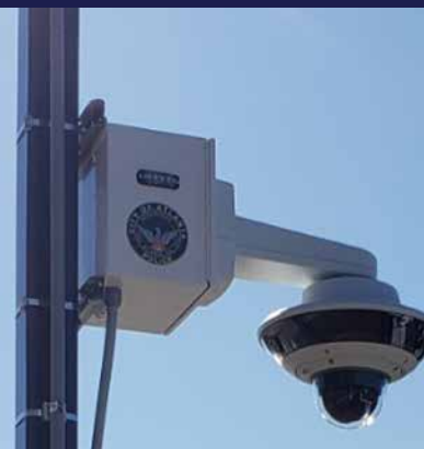
One of thousands of cameras throughout the City of Atlanta used to help fight crime and keep the city safe.
